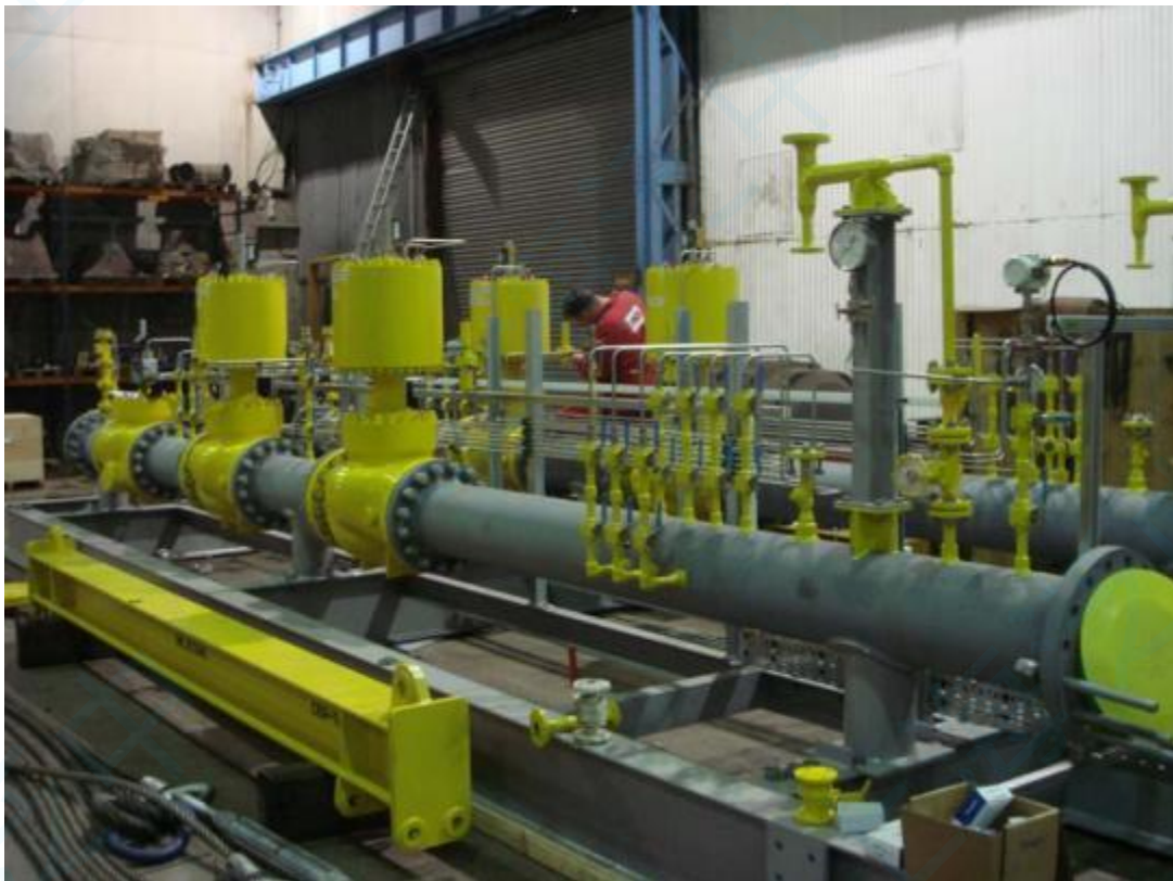
Fig 3.2.1 Installation of control valves series R100 in skid mounted pressure control and protection system
